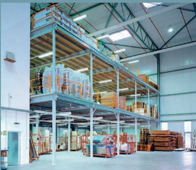
In the furniture storage. High support columns for the storage of bulky furniture parts. Storage platform with 3 floors, complete with railings, transfer station and sprinkler system from a single source.
