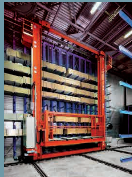
Rail guided twin mast storage and retrieval machine for order picking in a timber trade business
