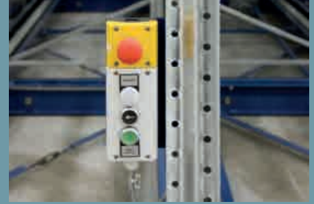
Electrical control of a traversing carriage
