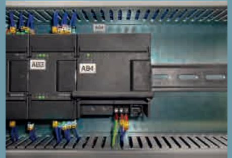
Electrical control modem for mobile rack systems
