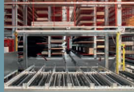
Transfer station from merchandise receipt into the automated warehouse
